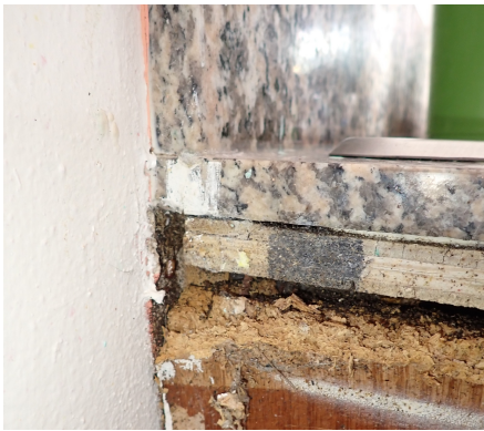
Figure 3. Structural deterioration plays a significant role in contributing to cockroach infestations. Damaged cabinetry, such as this decaying particle board, should be replaced or repaired. Photo credit: Josh Shoemaker
