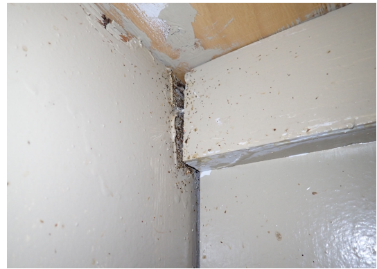
Figure 4. Unsealed gaps and cracks, like this cabinet corner, provide ideal harborage and travel routes for German cockroaches. Properly sealing these areas is a critical step in preventing infestations. Photo credit: Josh Shoemaker
