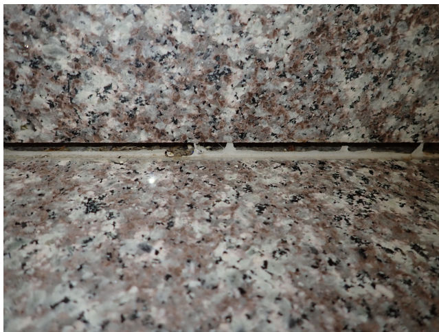
Figure 7. Unsealed gaps at the back of kitchen countertops, like the one shown here, provide cockroaches with easy access to hidden voids where they can shelter and reproduce. Additionally, trapped food debris and moisture within these crevices create ideal conditions for cockroach survival and can interfere with the effectiveness of bait treatments. Photo credit: Josh Shoemaker
