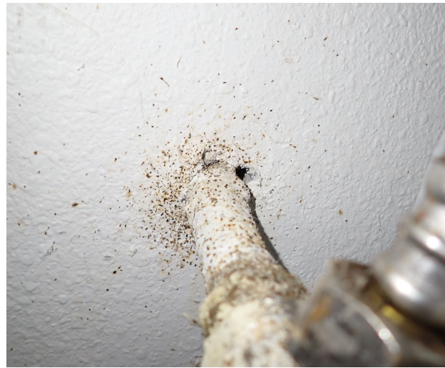
Figure 6. An unsealed plumbing entry point with visible German cockroach fecal material. Gaps like this provide cockroaches easy access to water, harborage, and migration routes between units, allowing them to thrive and reproduce. Photo Credit: Josh Shoemaker
